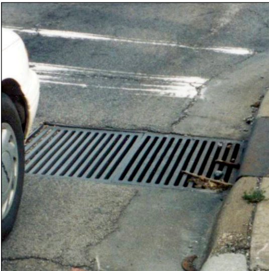
Example of bicycle unsafe grate with openings parallel to direction of travel
