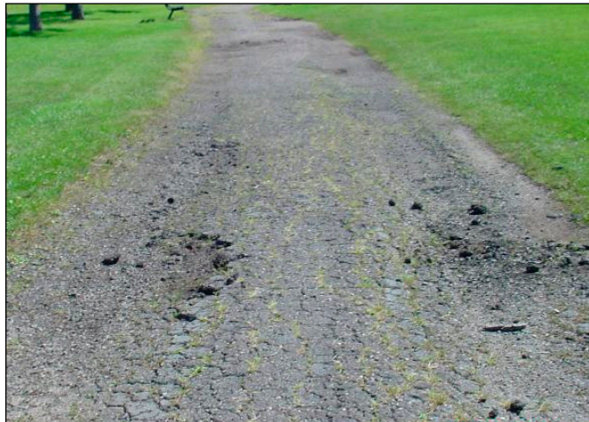
Figure 9-1: Deteriorated Shared-Use Path and Faded Markings
