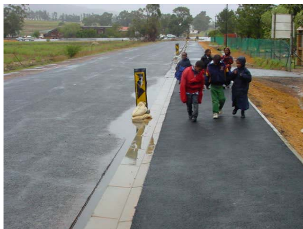
Figure 4-6: Water Ponding Along a Sidewalk
