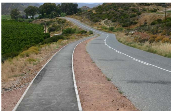
Figure 4-14: Unprotected Walkway too Close to the Road is Unacceptable
