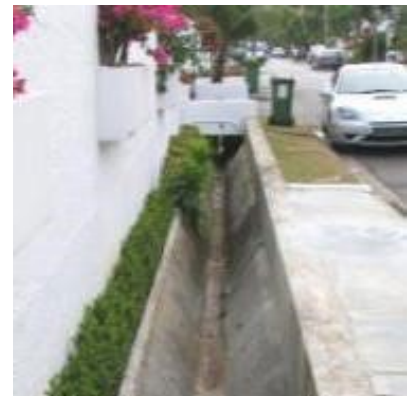
ABOVE: Open Composite channel drain beside footpath
