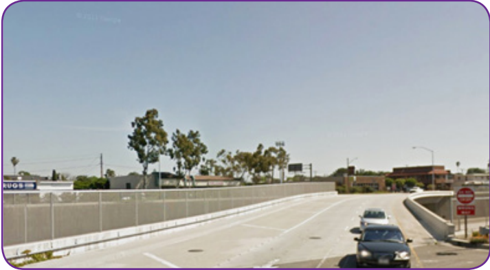
Figure 4-6 Looking south along the Fairview Road bridge over SR-55, wide striped shoulder visible
